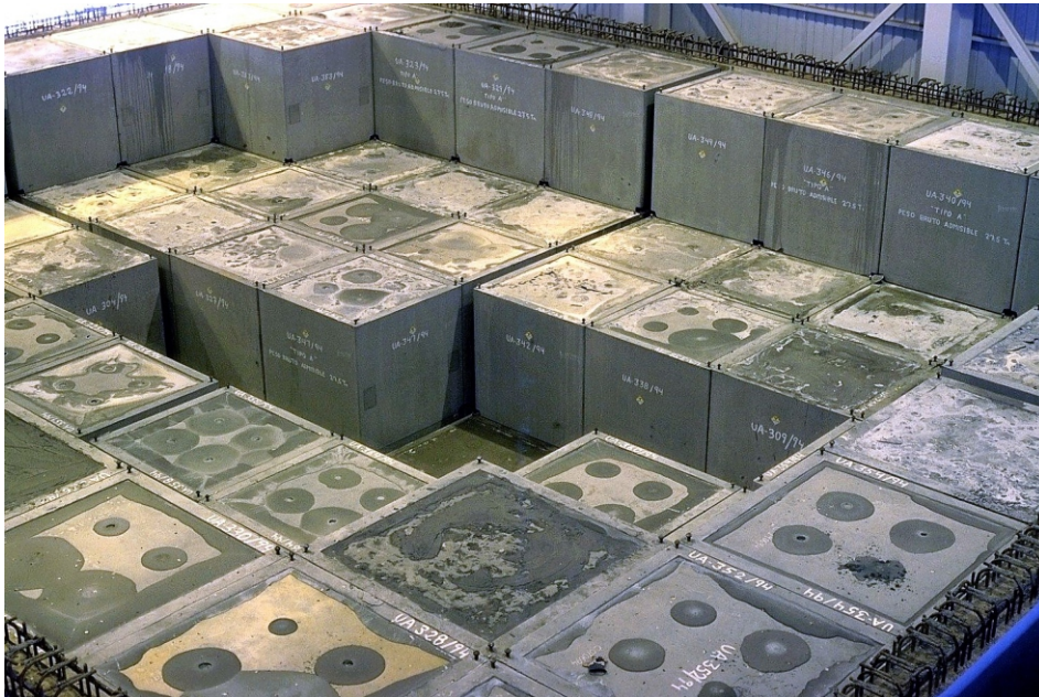
Detail of containers (disposal units) for the disposal of LILW in the storage cell at El Cabril.
