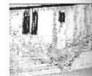
void inside of rubble bed.
