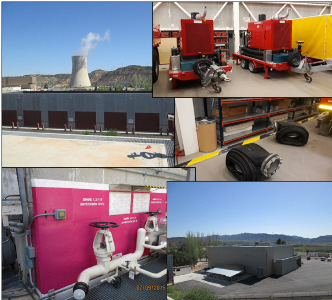
Storage building for portable equipment, portable water injection pumps, flexible hoses, quick-connect couplings for extensive damage mitigation strategies and the Alternative Emergency Control Centre at Ascó nuclear power plant in Tarragona, Spain.
